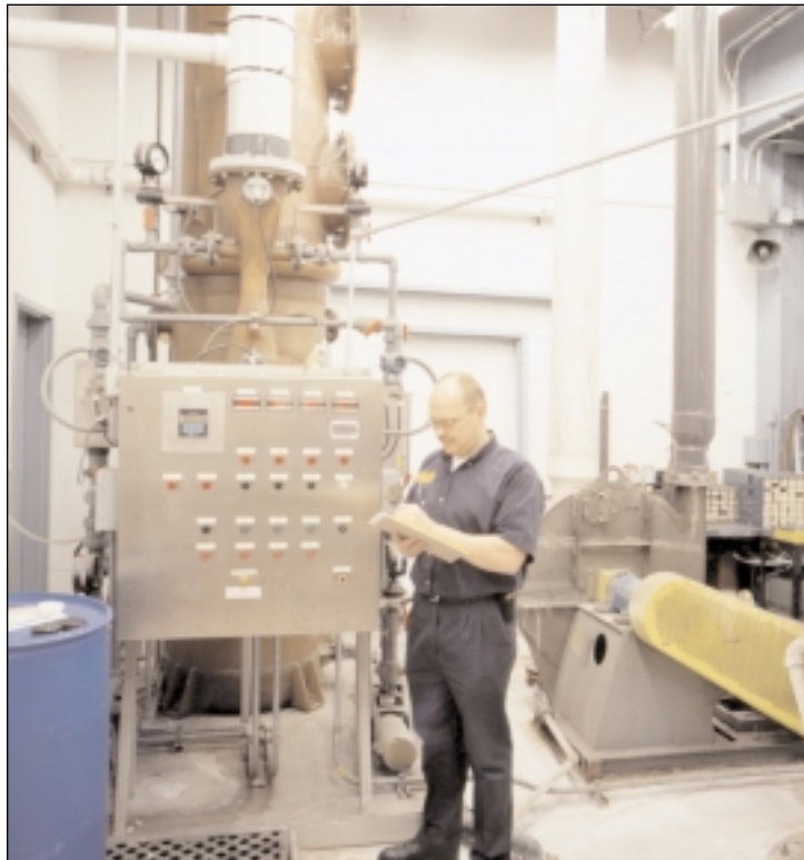
Jouko Tahvanainen, Facility Engineering Manager purchased their first Croll-Reynolds high energy fixed Venturi packed tower system in 1998.
